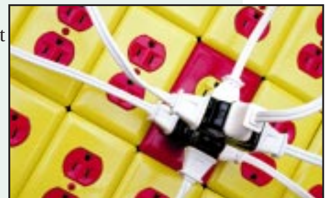
Overloads are a major cause of fires.
